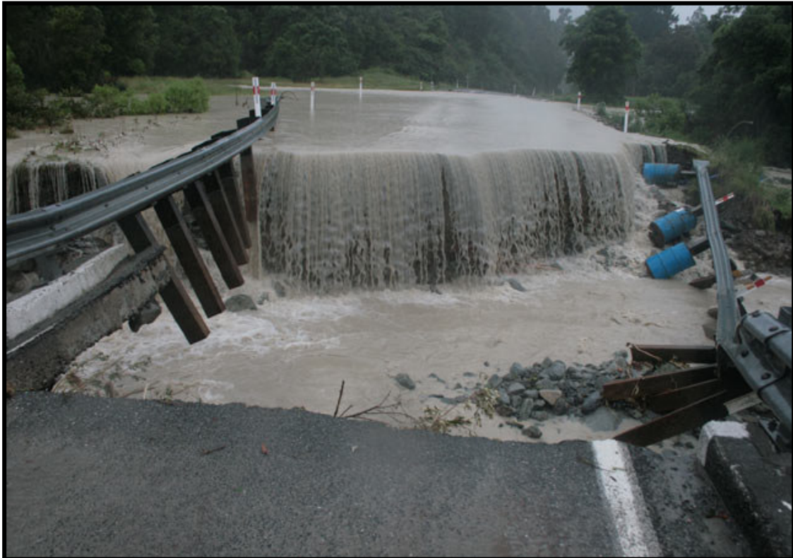
Wash out of state highway 73 at Kelly Creek. This is near the Taipo Rain gauge where 248mm of rain fell in 12 hours. Photo courtesy of NZTA
